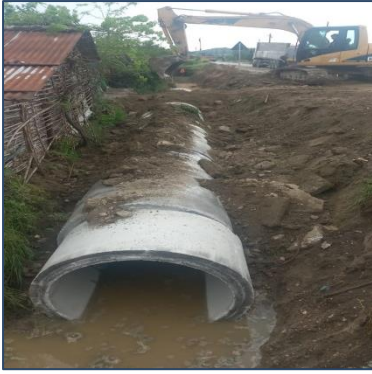
View of works being carried out to trench the drainage canal in Marinza village – July 2023
